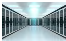
Large-scale server room
