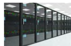
High heat density data center
